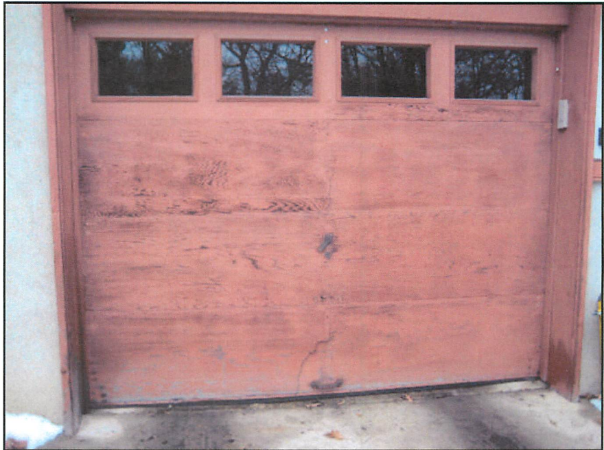
One door, Roll up. Roll up doors are the most common type. They travel on a metal track with counterbalance springs. Door is damaged, recommend replacement.
