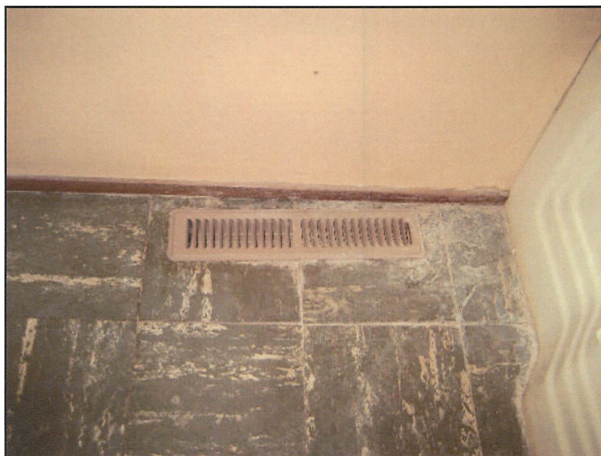
Staining on floor by tub and vent indicate past leakage. Water may have entered sub slab ductwork. See heating section.
